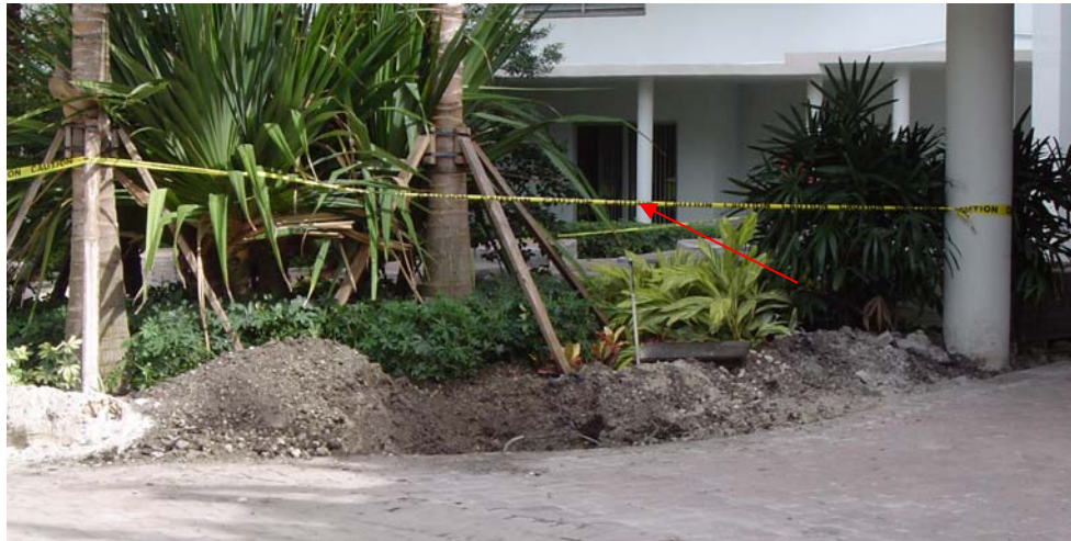
Plate 2. A safety tape (marked by arrow) placed from column to tree on an excavation.
