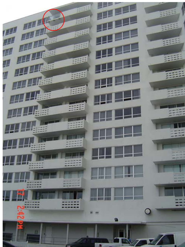
Plate 1. Work located on top floor for a 15-story building under renovation for new balcony railings
